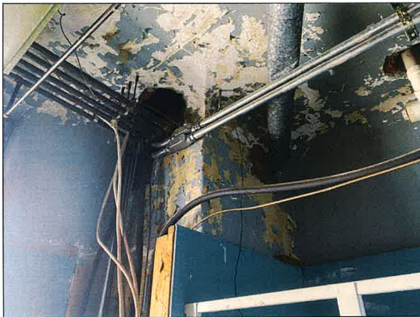
Photo 18: Building one; second floor peeling paint
