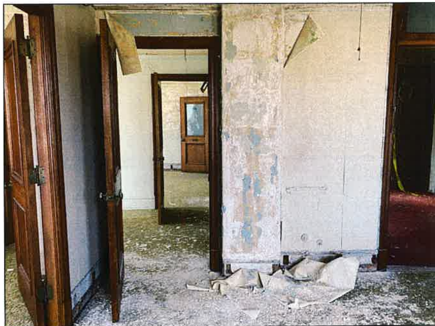
Photo 24: Building one; fourth floor peeling paint
