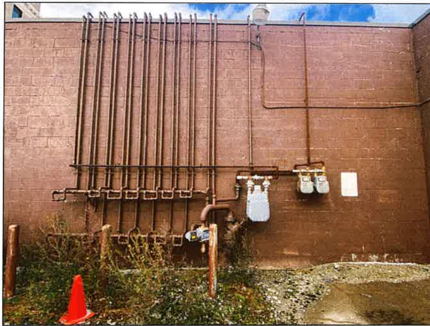
Photo 45: Building two exterior natural gas meters
