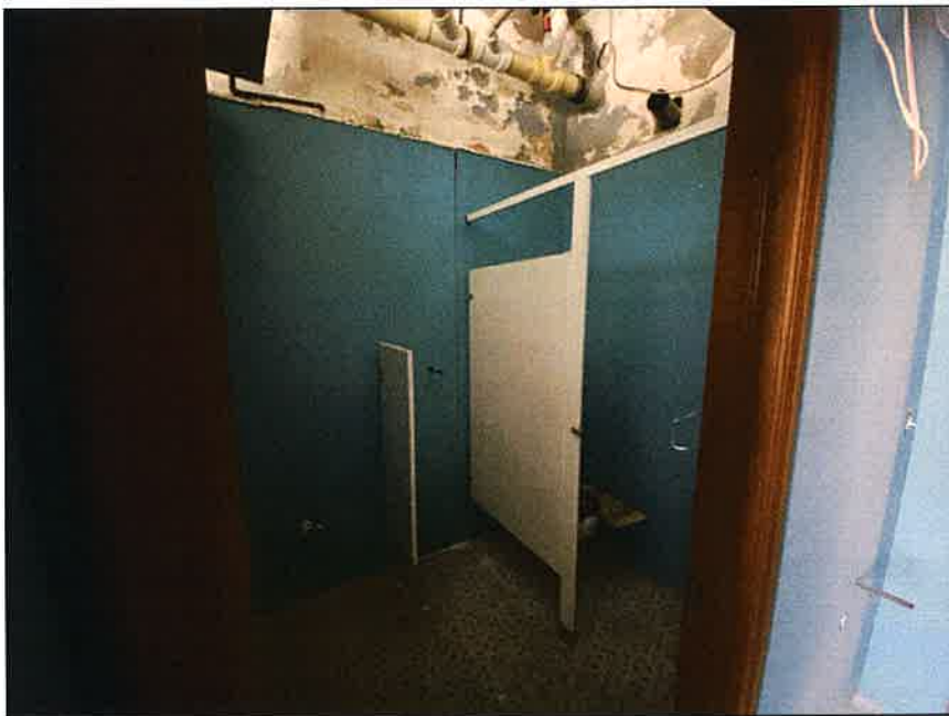
Photo 22: Building one; fourth floor bathroom
