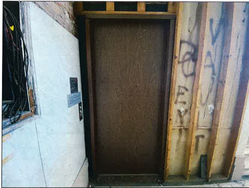
Photo 9: Building one; elevator
