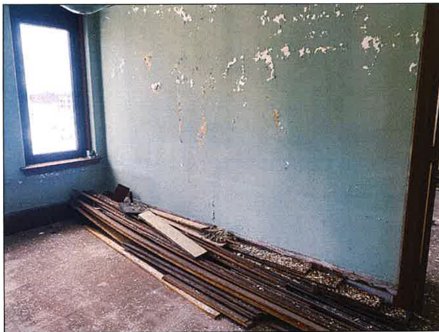
Photo 20: Building one; third floor peeling paint
