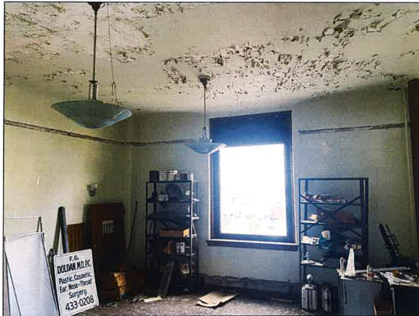
Photo 19: Building one; third floor peeling paint
