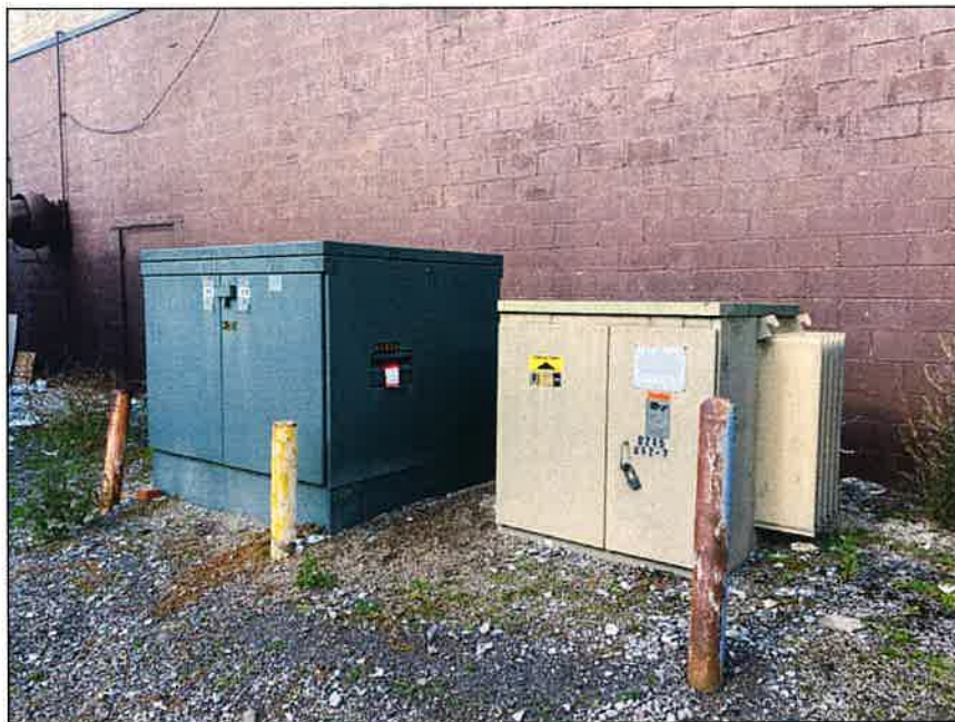
Photo 46: Two pad-mounted transformers
