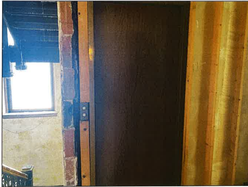
Photo 25: Building one; fourth floor elevator
