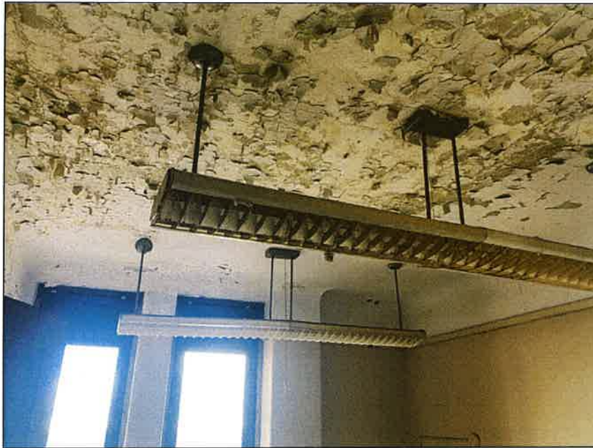
Photo 27: Building one; fifth floor peeling paint
