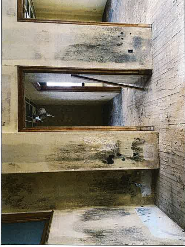
Photo 29: Building one; sixth floor suspect mold
