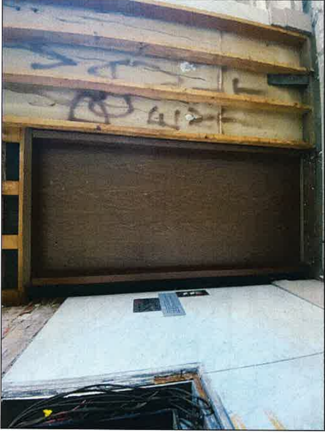
Photo 9: Building one; elevator
