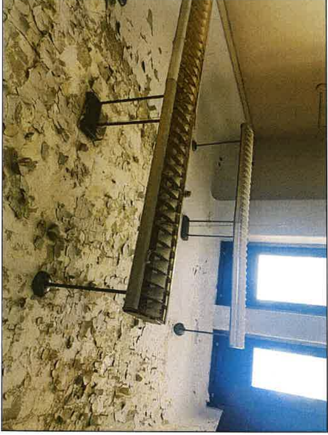
Photo 27: Building one; fifth floor peeling paint
