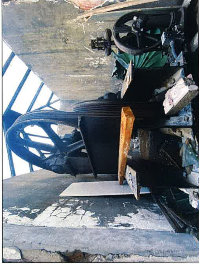
Photo 32: Building one; elevator equipment
