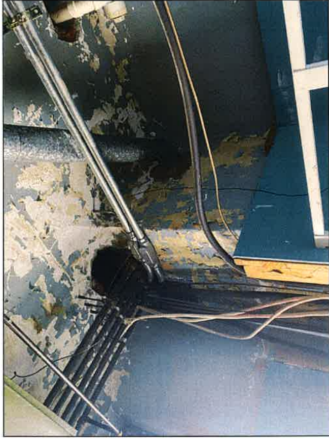
Photo 18: Building one; second floor peeling paint
