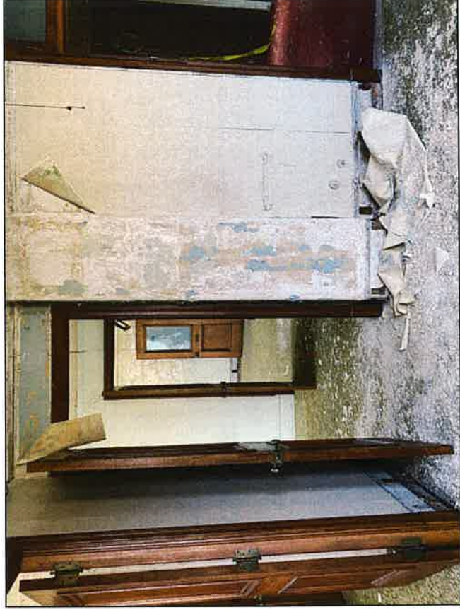
Photo 24: Building one; fourth floor peeling paint
