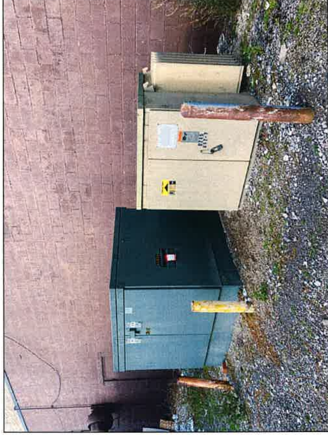
Photo 46: Two pad-mounted transformers
