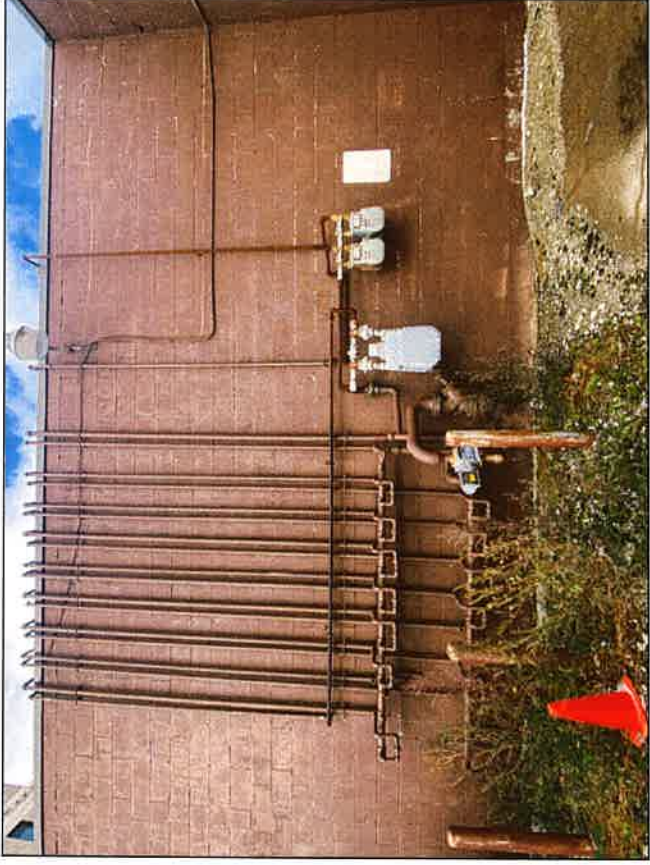
Photo 45: Building two exterior natural gas meters
