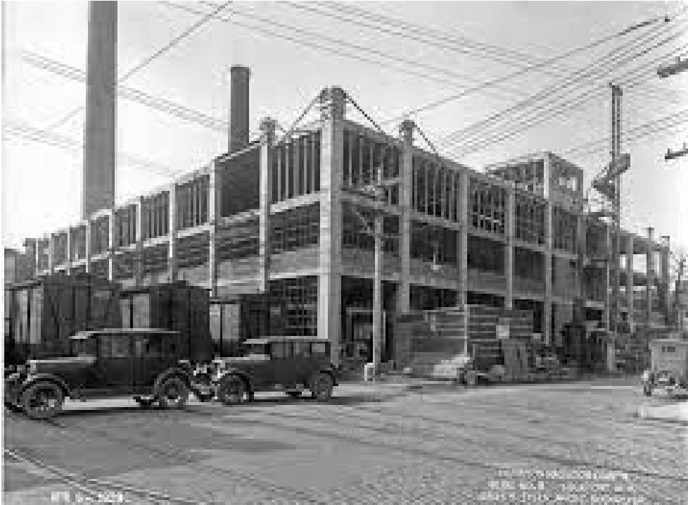
Harrison Radiator Building #3 under construction April 1929. View is looking SW, intersection Walnut & Elm St., Lockport NY. 2nd photo as it looks today.
